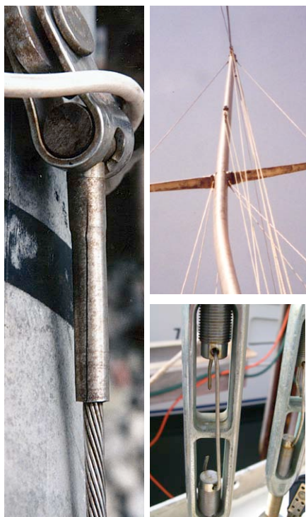
Left: A cracked swaged fitting like this can bring the whole rig down. Top right: A stay broke on this mast in light winds, but fortunately the rig stayed up. Bottom right: Replace cotter pins with welding rod to avoid snagging lines.
